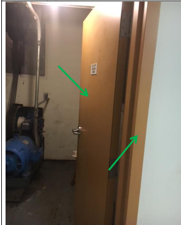
Photo 3: Orange paint on metal door and door frame is not lead containing.
