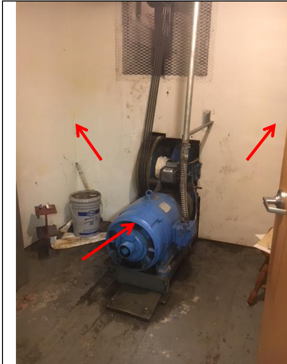
Photo 1: Drywall joint compound on walls in the Elevator Machine Room is asbestos containing. Blue paint on metal elevator machine equipment is lead containing.
