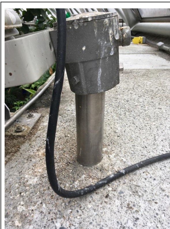
Photo1: Perimeter Lighting - Close up
