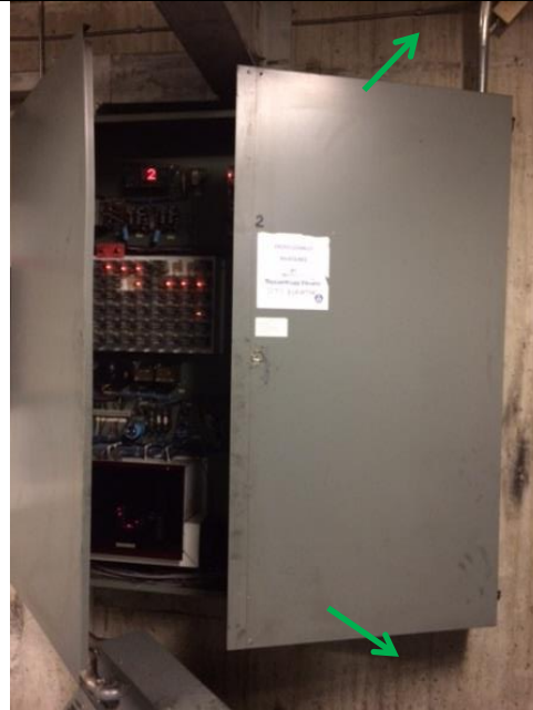
Photo2: Unpainted concrete walls throughout elevator machine room.
