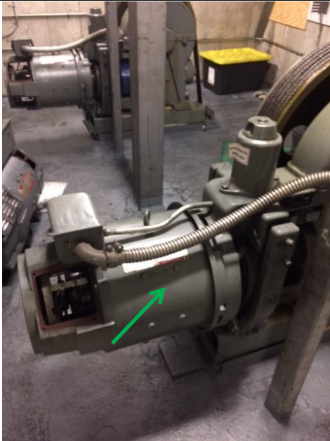
Photo 1: Grey paint on metal elevator machine equipment in elevator machine room is lead containing.
