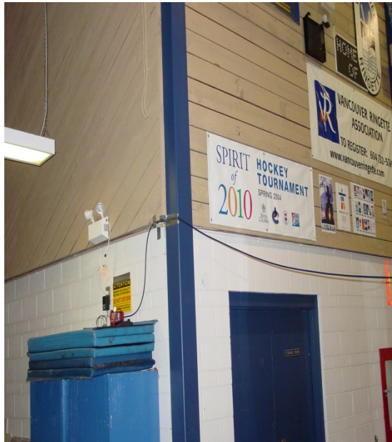
Photo 4: Interior Cinderblock Walls may contain Vermiculite Insulation within.
