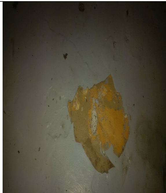
Photo 3: New grey paint coat on multiple layers of old paint - Lead based paints.
