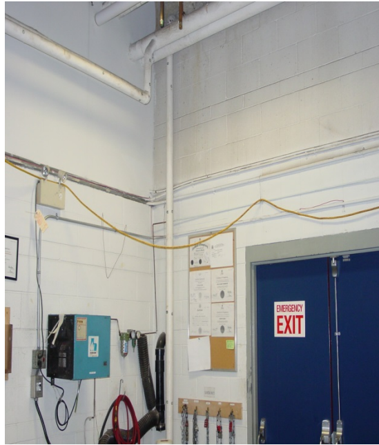
Photo 2: Painted Mud on Drywall walls do contain asbestos
