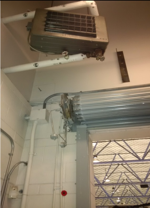
Photo 1: Hard Mud Elbows do contain asbestos.
