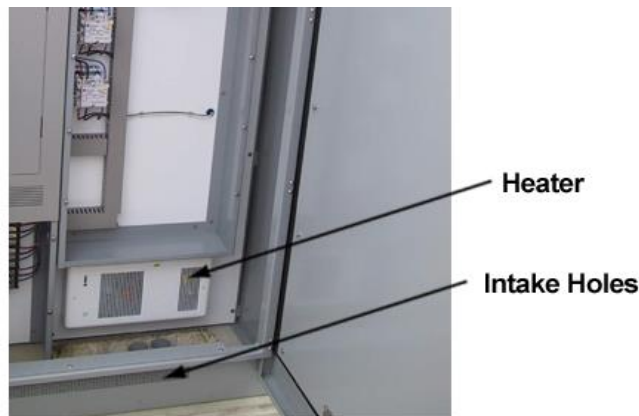
Figure 4 - Heater and Intake Holes
