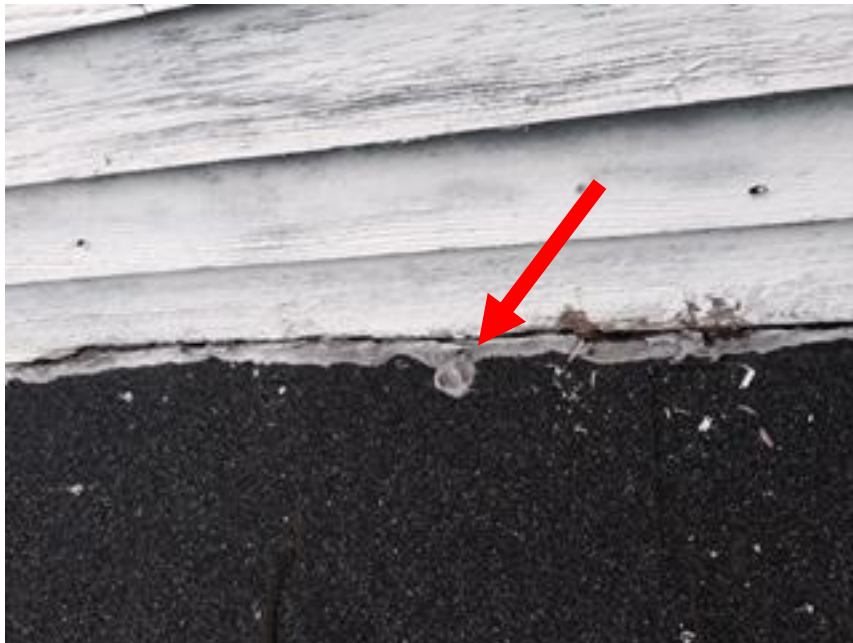
Photo # 2 – Asbestos-containing mastic
