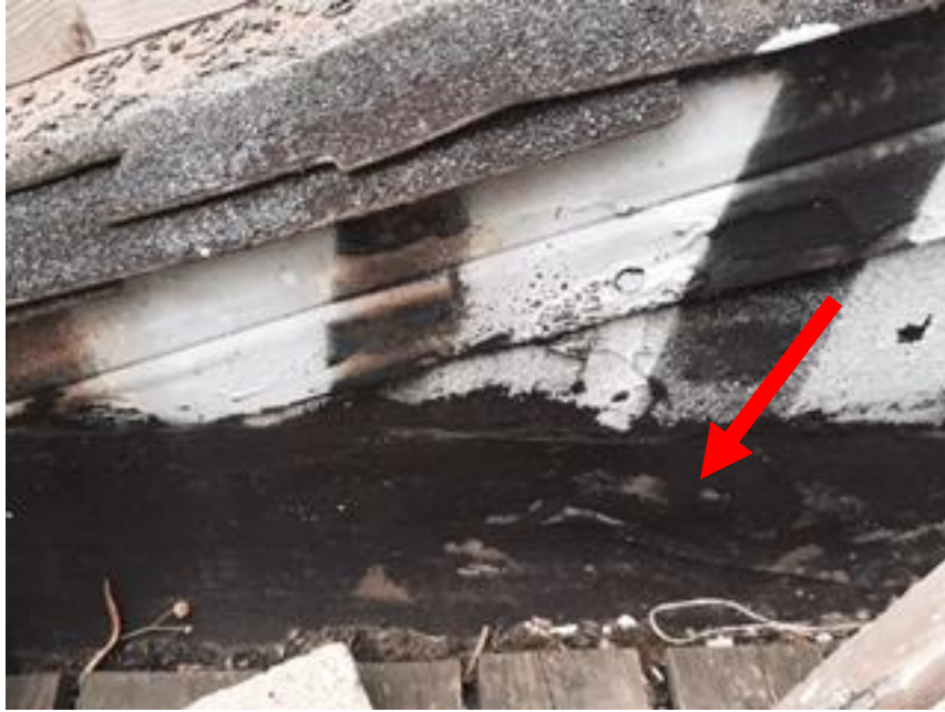
Photo # 1 – Asbestos-containing mastic
